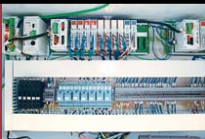
New Electrical Panels—UL Listed
